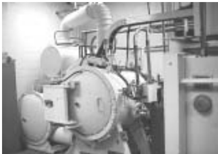
• High velocity quench vacuum heat treatment furnace
